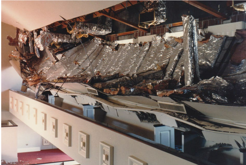
The collapsed ceiling of 1962
